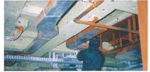
天井部防火 Fire resistance treatment and heat insulation of ceiling area
