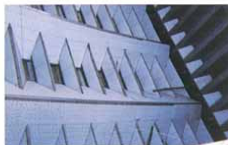
石炭運搬船 倉内ライニング工事 Lining work in cargo area on coal transport ship
