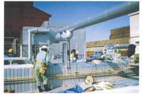
集塵装置上部保温工事中 Heat insulation of upper part of dust collection system
